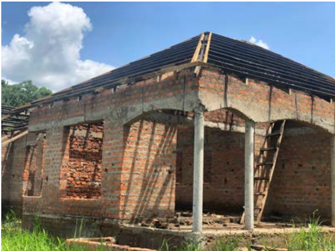
Progress photo of our children's home with roofing timbers during phase IV (the roofing)
